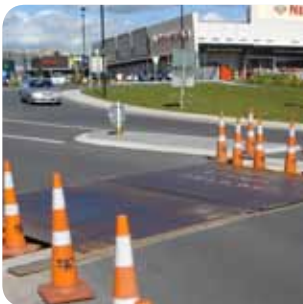
Road works, uneven surfaces and metal plates can all be hazardous in certain situations
